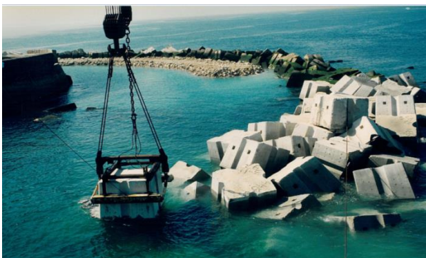
Figure 7: Transportation and laying of the rockfill layer and Antifer cubes in the surrounding of the Fortress. Photo courtesy, Eng.º Lopes de Castro.
